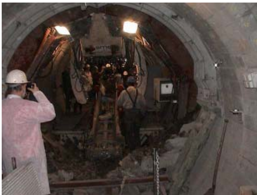
The crucial moment: the access of the tunnelling machine to the underground labo HADES
