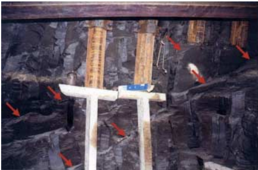
Figure 5-25: Second shaft: slip planes and fractures observed during excavation of the starting chambers. The upper picture shows a fallen block in the south starting chamber due to a circular (vis-à-vis the centre of the second shaft) slip plane. The below picture shows the side wall of the same starting chamber displaying cross-sections of two of the encountered fractures (average dip was 35° towards the centre of the shaft).
