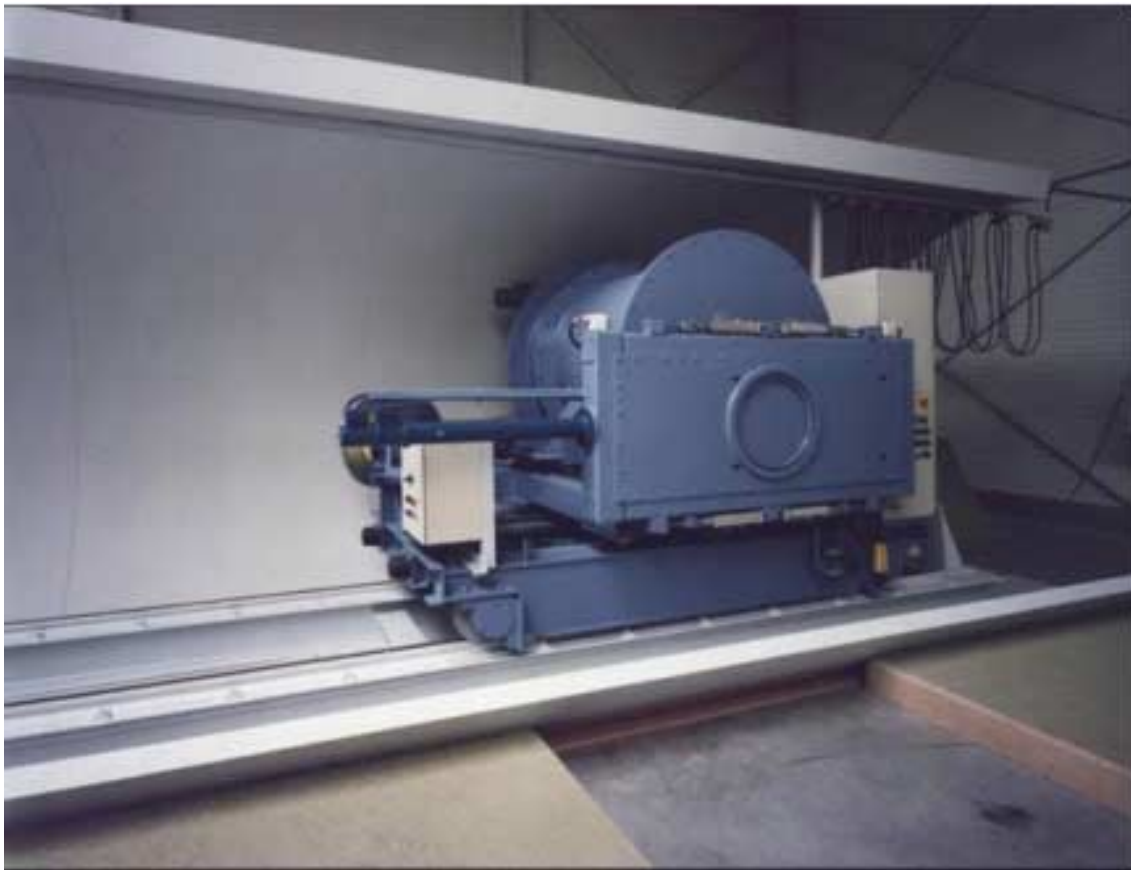
Figure 6-5: Transfer wagon (PRACLAY demonstration hall).
