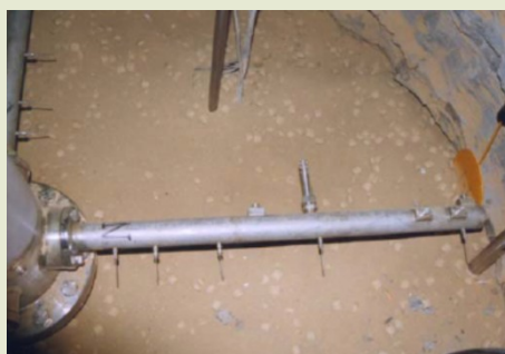
Figure 69 – RESEAL test: tube instrumented for total and pore pressure, relative humidity and temperature measurements (RESEAL II, 2009).
