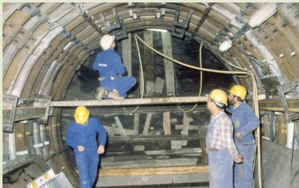
Fitting the lining at the end of the second gallery, called "Test Drift"
